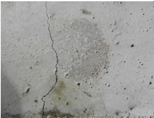
Fig. 6: Cracking on top compression face of beam
