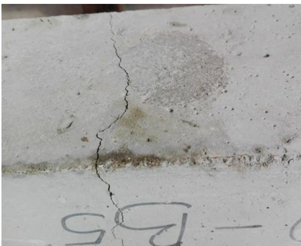
Fig. 7: Crack pattern at ultimate failure
