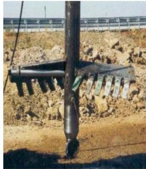
Fig. 7. Installation of lime column in the field using Trevimix method (Paviani and Pagotto, 1991)
