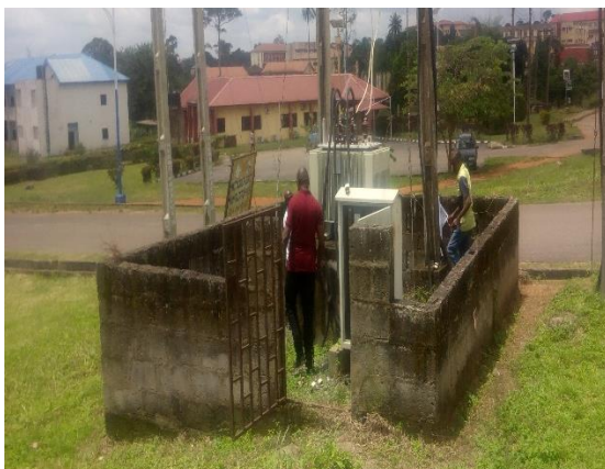
Figure 3: Typical substation in the study Area
