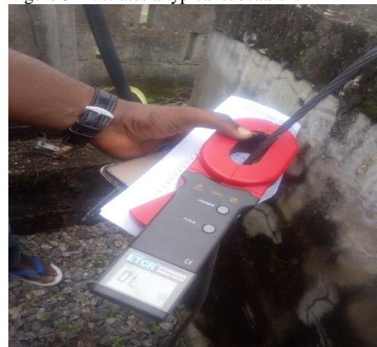
Figure 2: Clamping of Earthing Conductor Using ETCR 2000 Series Earth Ground Meter
