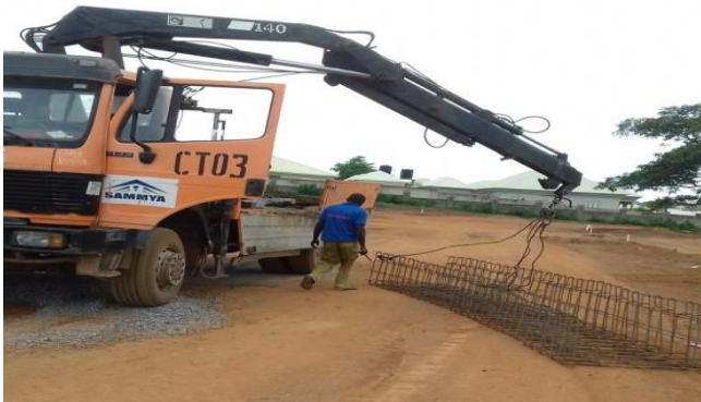
• Plate 1: Mobile crane used in the lifting of reinforcements on Market Site
