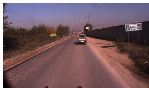
Figure 3 Road SH2 Tiranë–Krujë, x 492.1622,y 46.79,km 8 + 66 m
