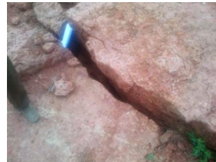
Plate 5: Showing evidence of subsidence (black line showing line of fault while the orange line shows extend of displacement)
