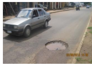
Fig. 3a: A typical pothole
