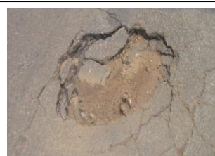
Fig.3b: Potholes surrounded by alligator cracks
