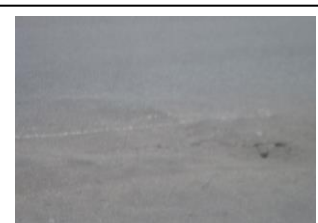
Fig.3c: Low severity longitudinal cracks
