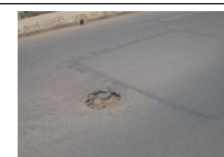
Fig. 3d: A patch next to a pothole
