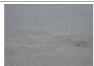
Fig.3c: Low severity longitudinal cracks
